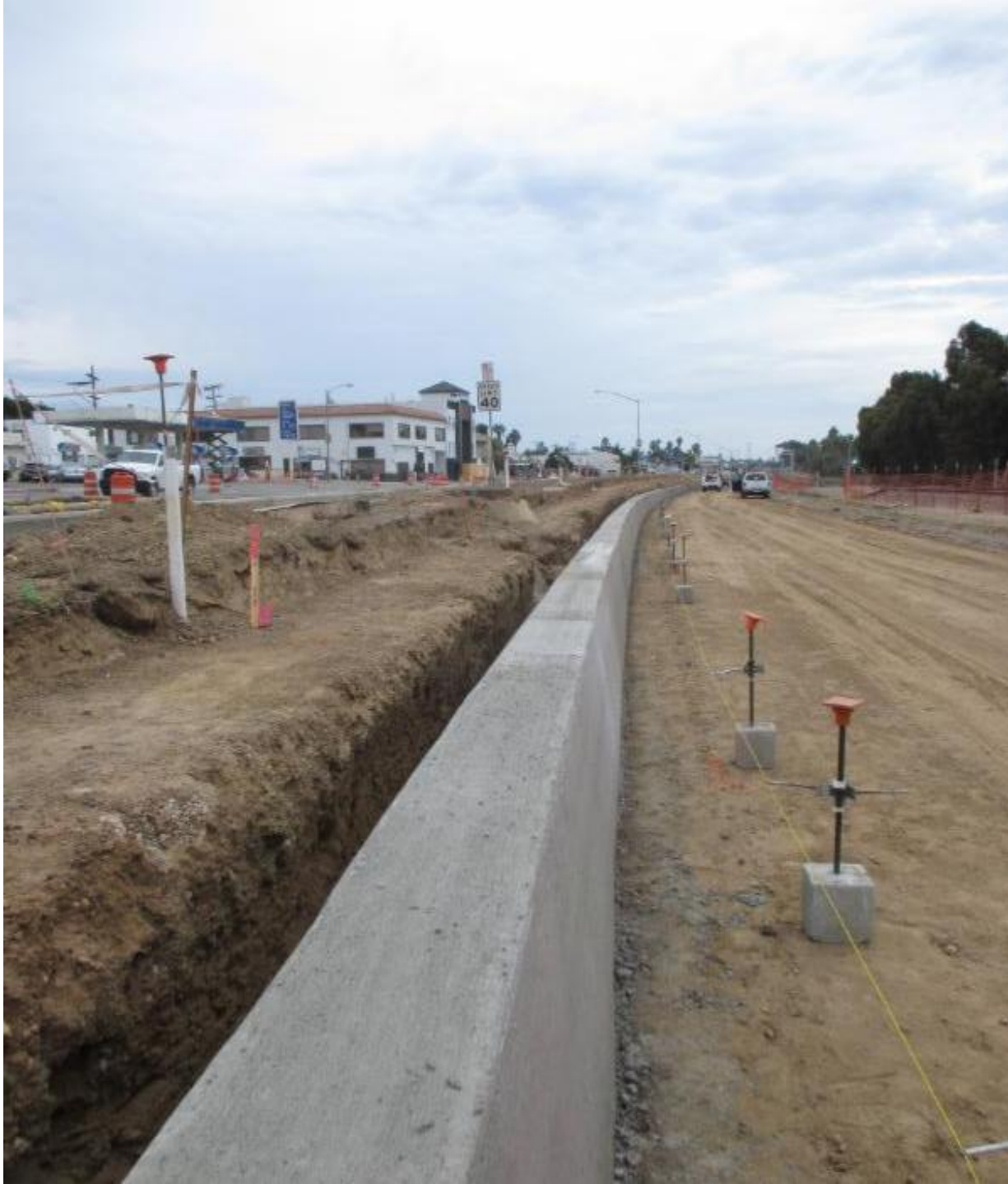
The ballast curb recently installed by CEI using the slip forming process.
