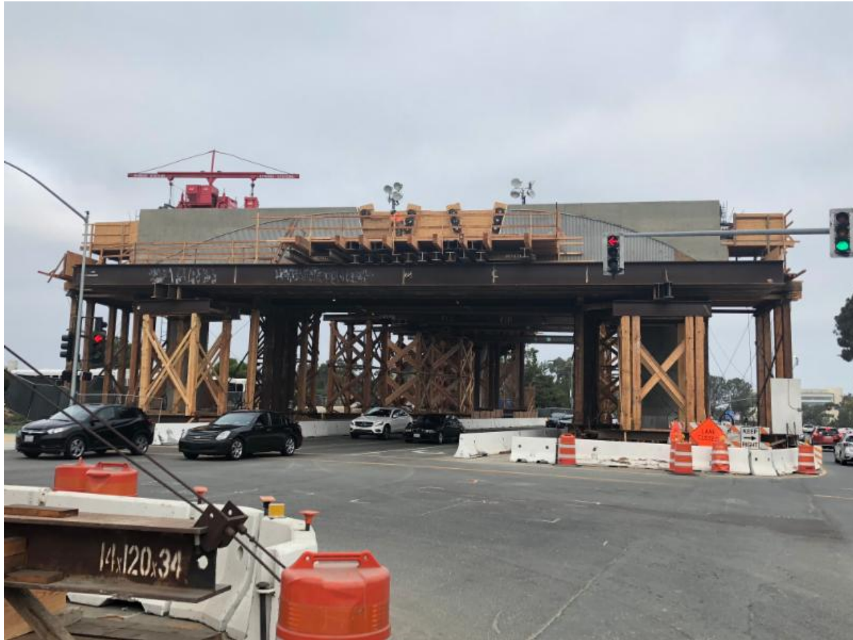
South side of the outrigger at the intersection of Genesee Avenue and Regents Road.
