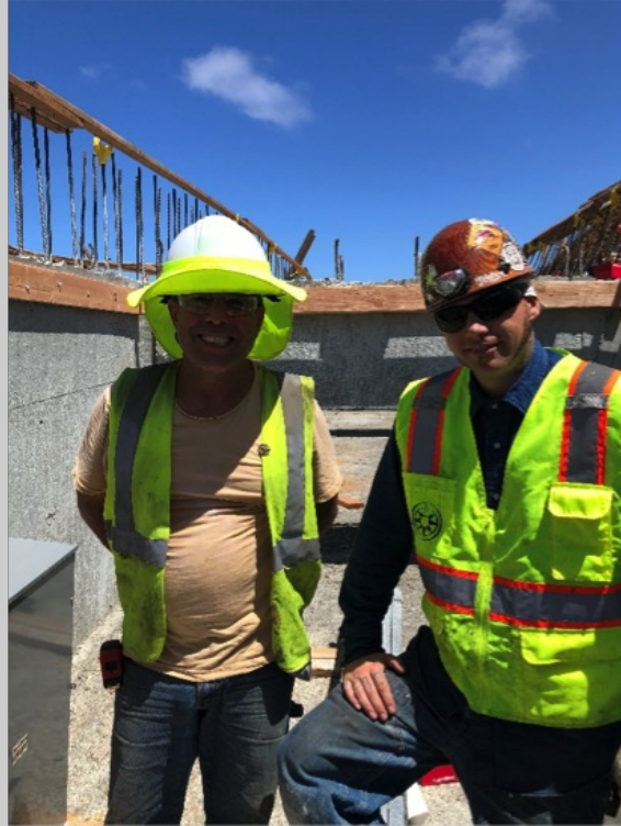
Renee (left) and Mike with Paradigm Mechanical Corp., taking a moment to explain the plumbing installation at Pepper Canyon.
