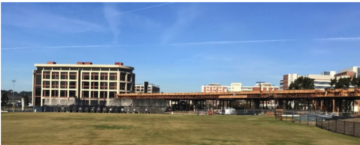
A section of the Genesee Viaduct that will pass through a UCSD Recreational Field.
