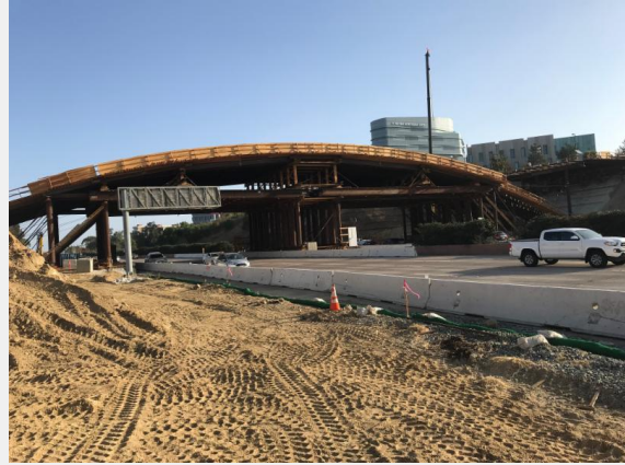
View of the Gilman Bridge falsework showing the profile that suggests its classification as an "arch" bridge.
