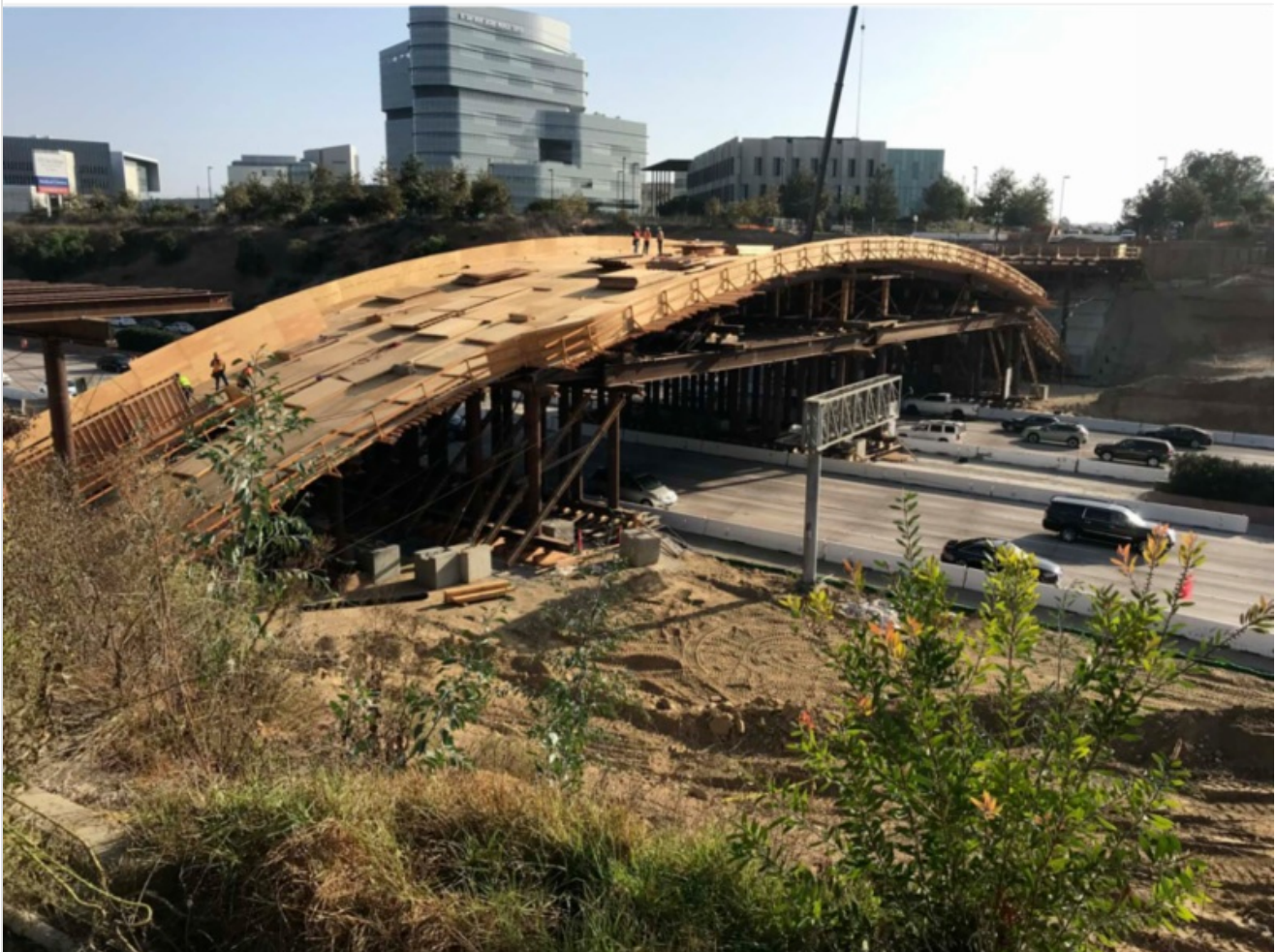
MCTC setting up for the next X Games? No...this is actually the falsework for the construction of the Gilman Bridge. (View facing east.)
