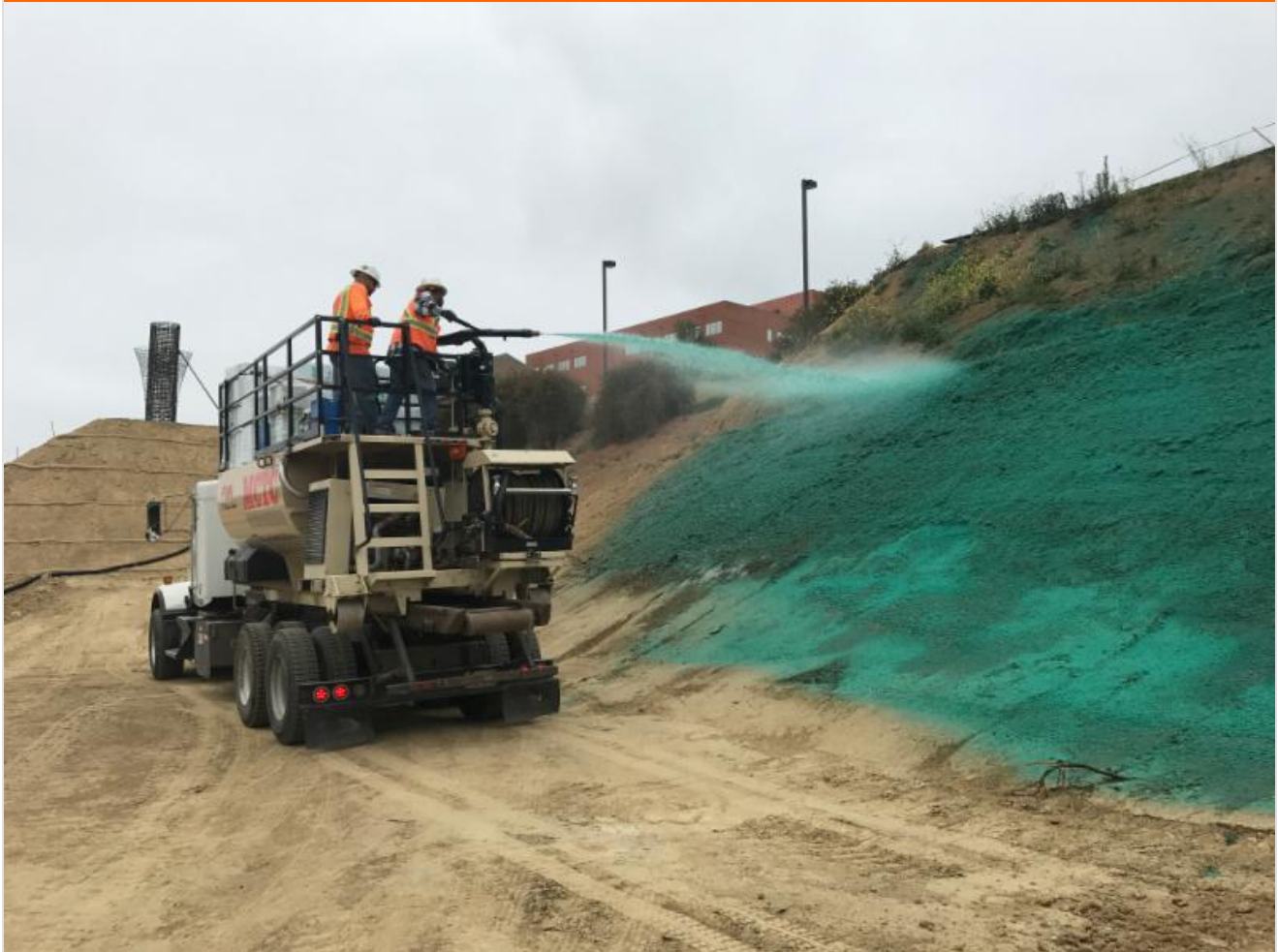
Hydro-seeder in action (used to spray mulch and seeds on disturbed soil to minimize erosion)
