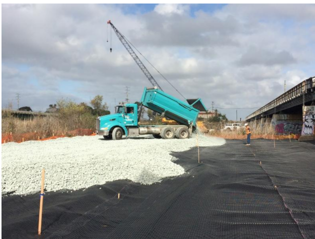
Bert W. Salas, Inc. building access road at San Deigo River Bridge
