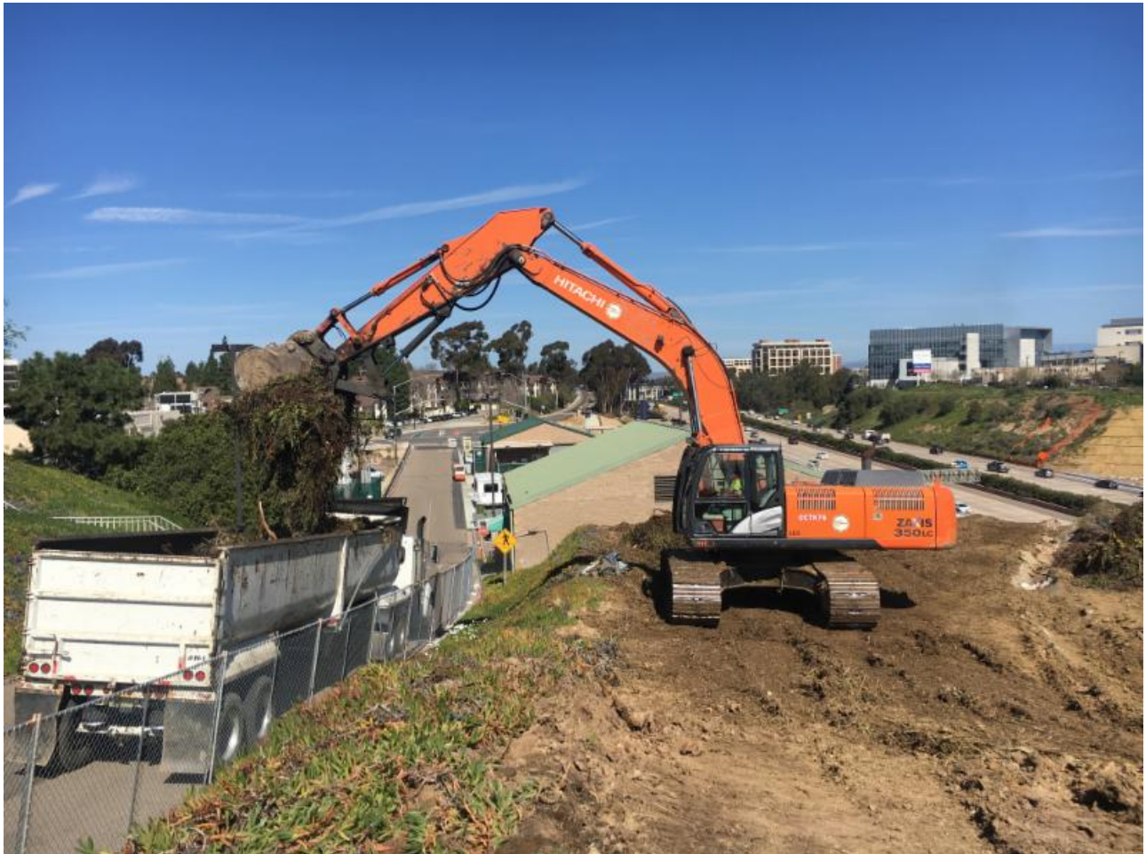
CGO (a DBE sub-contractor) clearing and grubbing on the north end of the Mid-Coast Corridor Project
