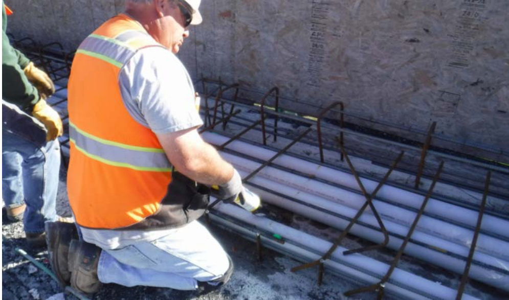
Moor Electric performs current testing on steel rebar prior to a concrete pour.
