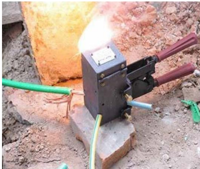
A mold is clamped down around the wires being joined together, then a special powder is used to create an exothermic reaction which produces enough heat to melt the metals together.
