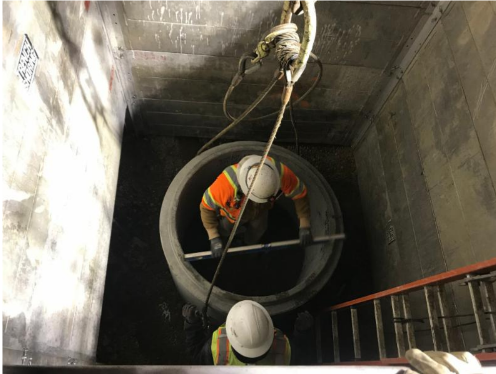
MCTC workers coordinate with Paradigm Mechanical to install a sump pit at the base of an elevator shaft.
