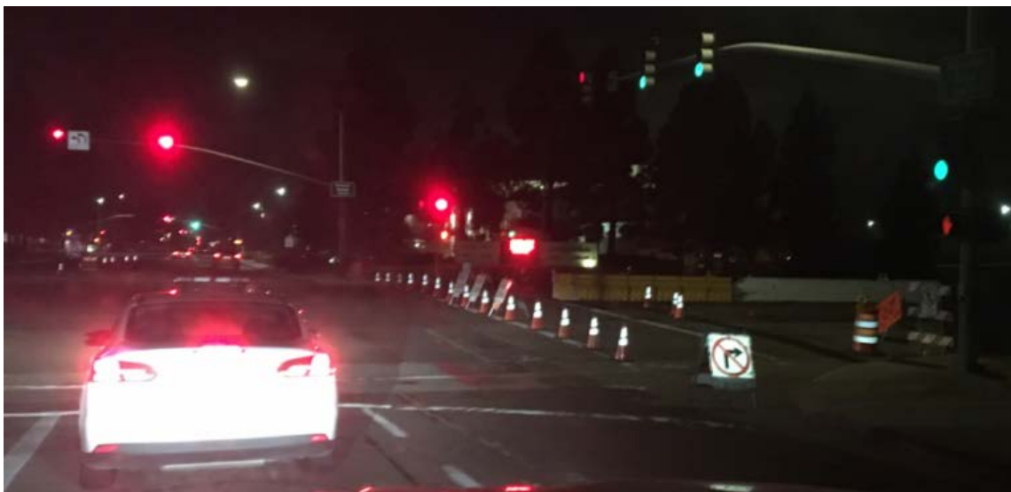
View of MCTC traffic control (i.e, cones, signs and barriers) placed by MCTC subcontractor, E-Nor Innovations Inc., to safely direct traffic around an overnight Project road closure.
